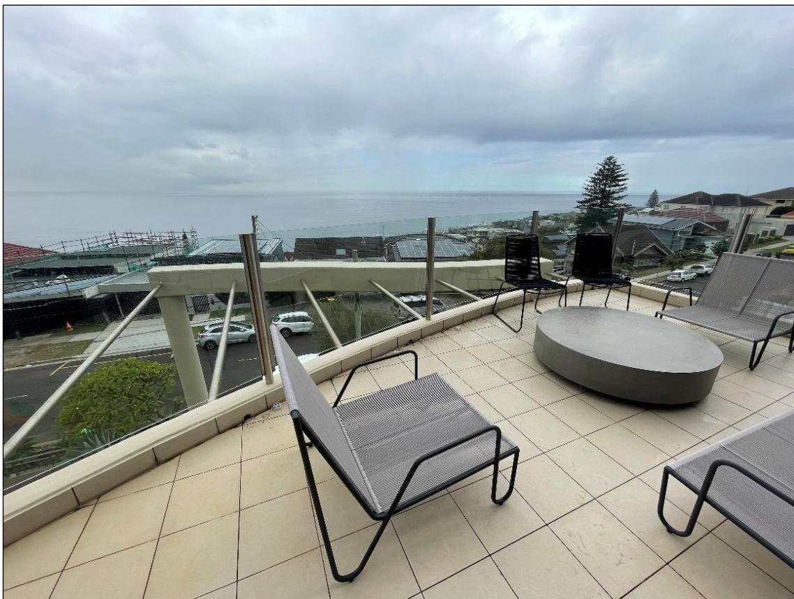
Figure 3: Balustrade proposed for replacement – area of height limit exceedance
