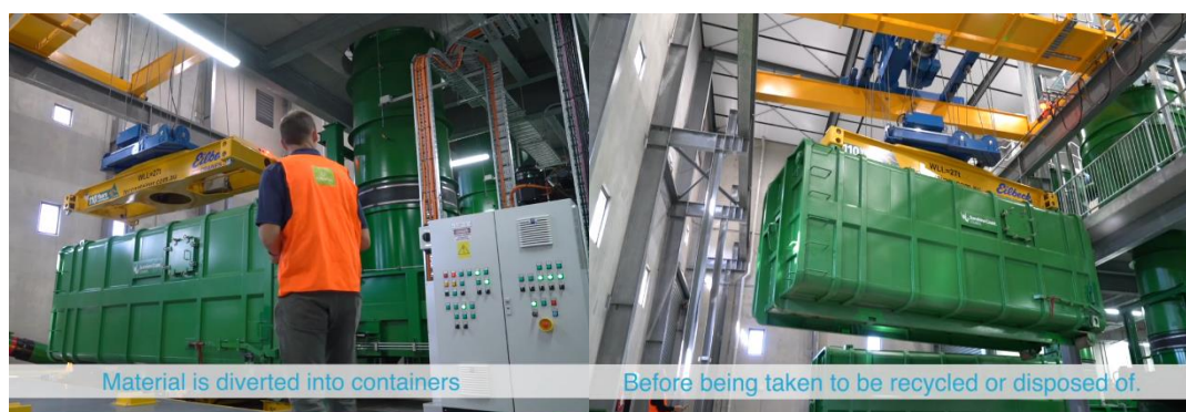
Figure 4: The Maroochydore AWCS collects waste is transported to recycling facilities and stored in container, negating the need of vacuum trucks.
