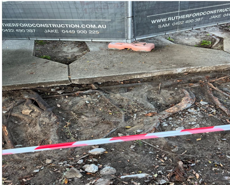
Tree roots in the driveway
