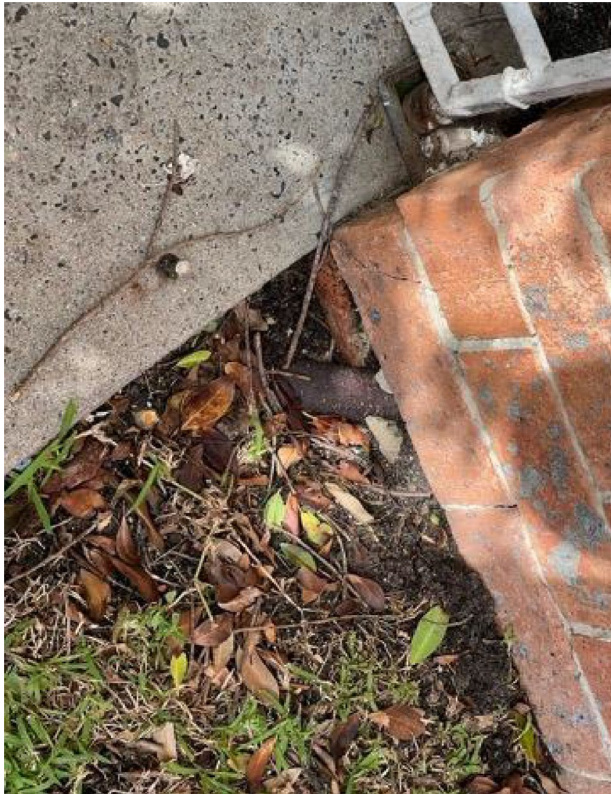
Tree roots inside fence and damage
