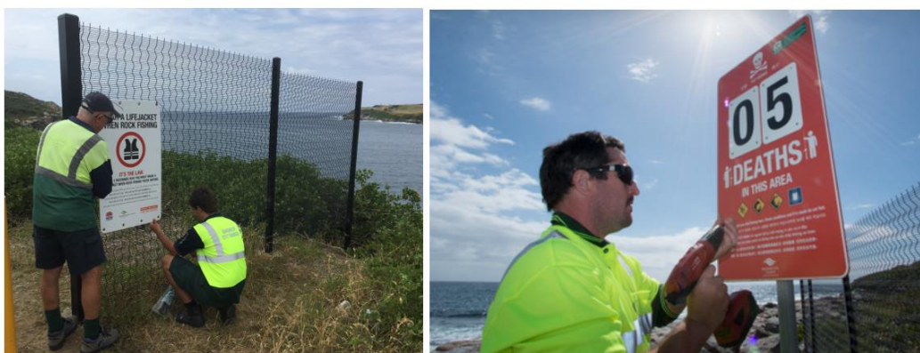
Council staff installing lifejacket signage (left) and shock signage (right) showing the number of deaths in the locality.
